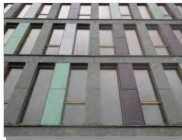
Figure 6: PV Modules in the Façade
