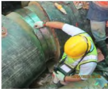
Figure 11: Insulation of DCS Pipelines
