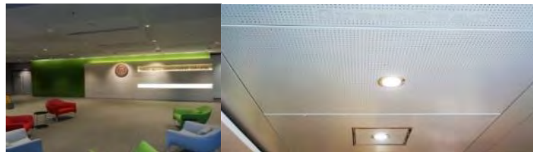
Figure 4: On-site overview of chilled ceiling air conditioning system
