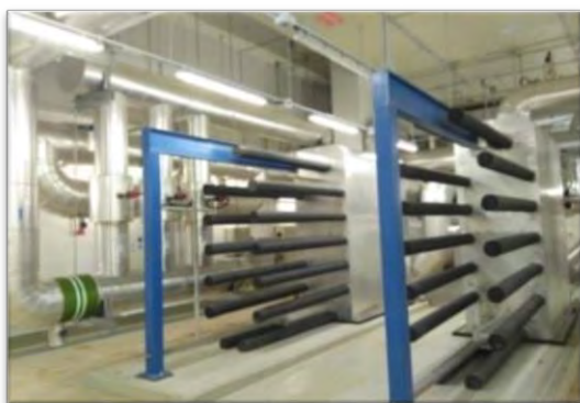
Figure 13: The heat exchangers in DCS substation
