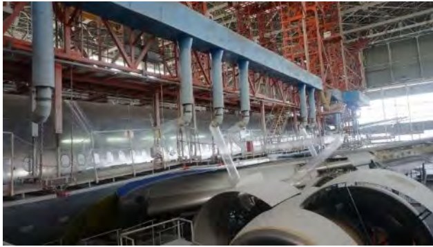
Figure 2.2a: Chilled air supply at Bay area
