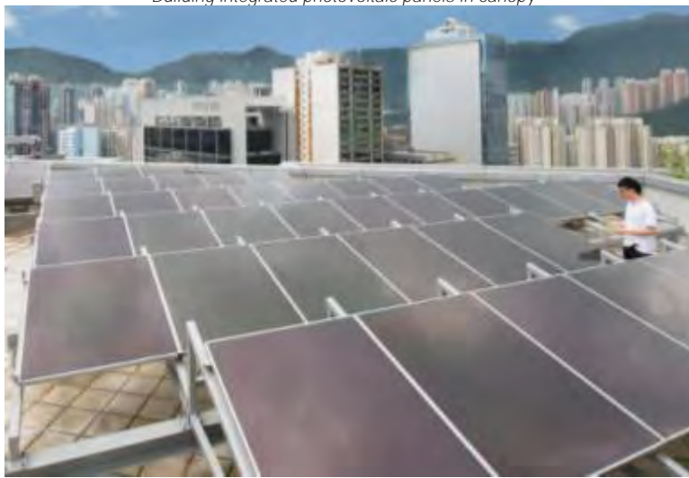
Photovoltaic panels on upper roof
