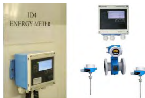
Figure 14: The energy meter in consumer building
