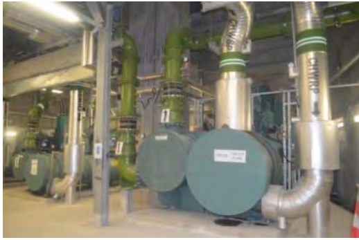
Figure 6: The installed 1.4MW and 4.3MW chillers at the basement floor of North Plant
