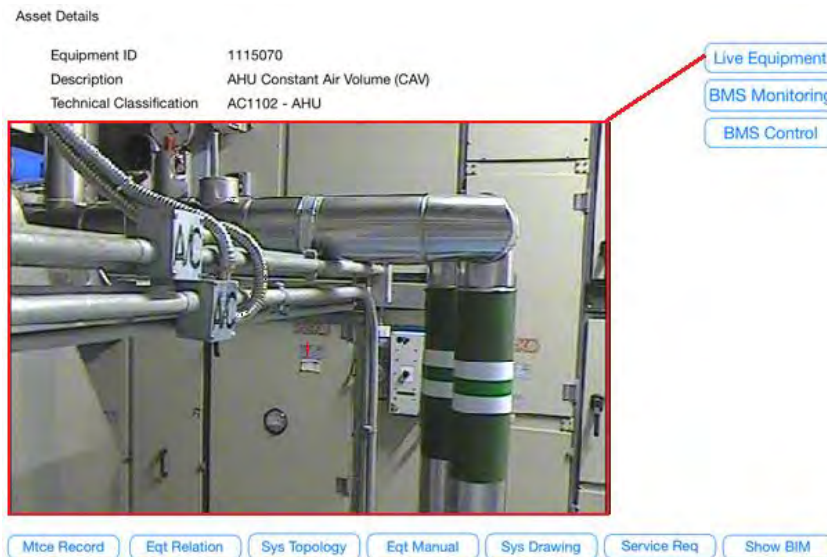
Figure 5: The live feed of a wireless camera in the BIM-AM system
