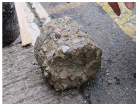
Figure 3: Core taken from early site trial indicating significant cementation occurred in recycled sub-base layer
