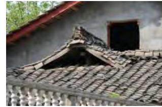
Figure 10: The hole on the gable structure
