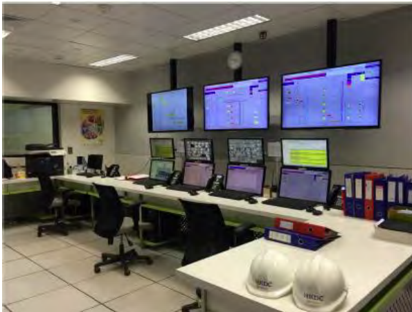
Figure 15: The control room in North Plant
