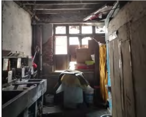
Figure 90: One water room.
