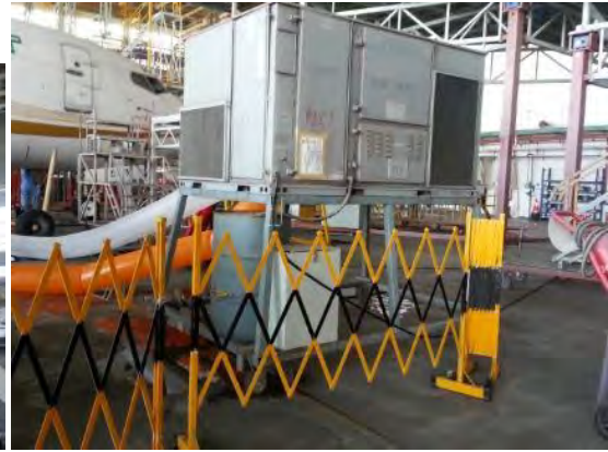
Figure 2.2b: Mobile air conditioning vehicle
