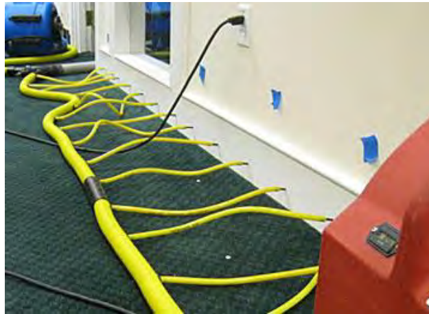
Figure 5: Drying wet wall with presence of insulation
