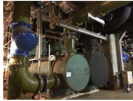
Figure 7: The installed 17.5MW chiller at the basement floor of South Plant
