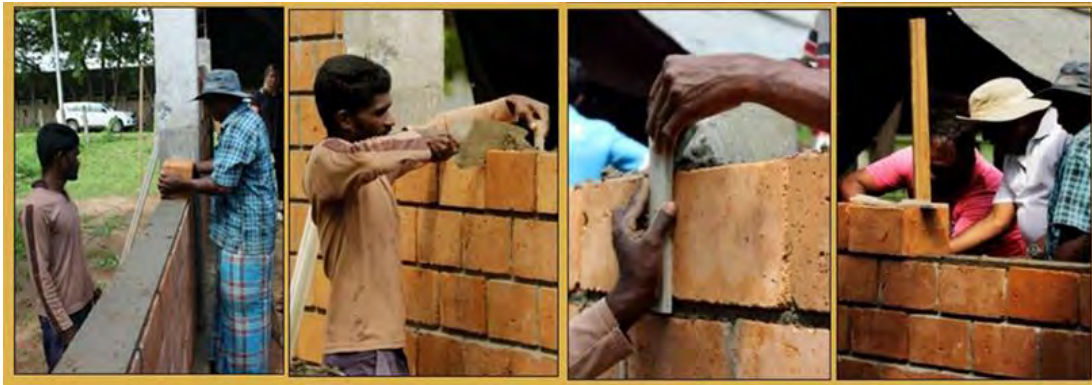
Figure 3: Easily handled simple tools & techniques were introduced to maintain the quality of construction
