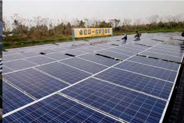
Figure 2: Taiwan's first floating solar power station
